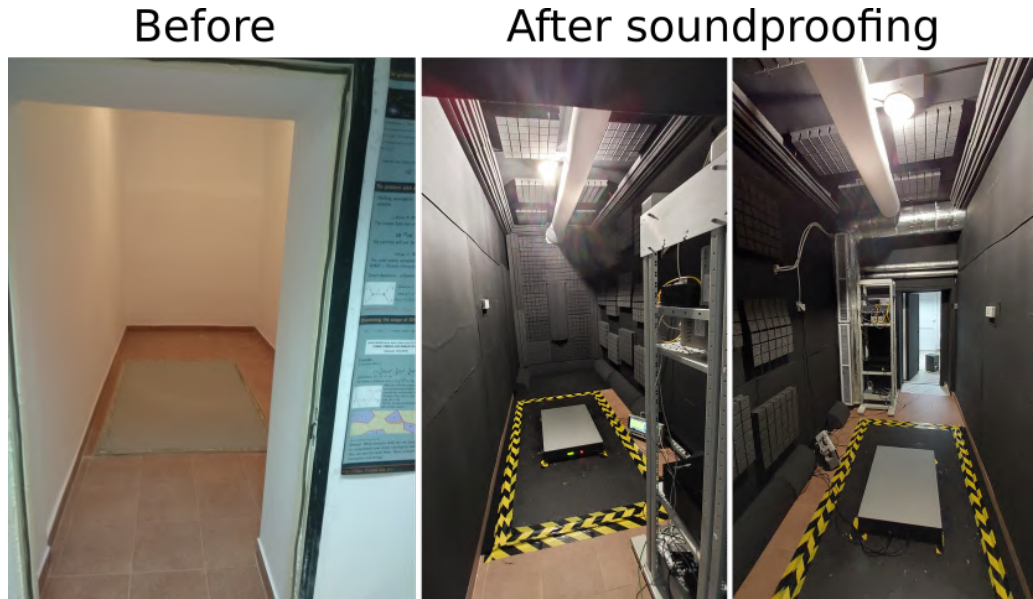
Figure 4.12: Cavity's room before and after acoustic insulation. The black-taped rectangle in the right photo represents a separate foundation on which the Table Stable TS-300 rests during the measurements.
